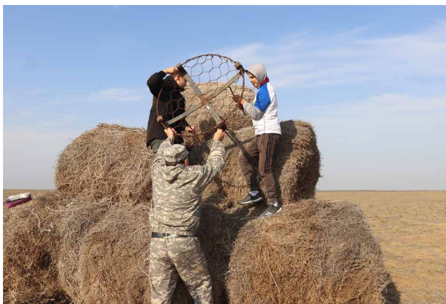
Installation of a frame for a raptor to nest on. Photo: Tatyana Gaydukova
